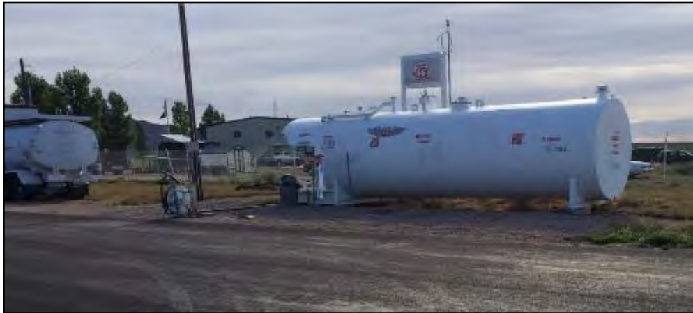
FIGURE 4-10 – 100LL AVGAS STORAGE TANK
